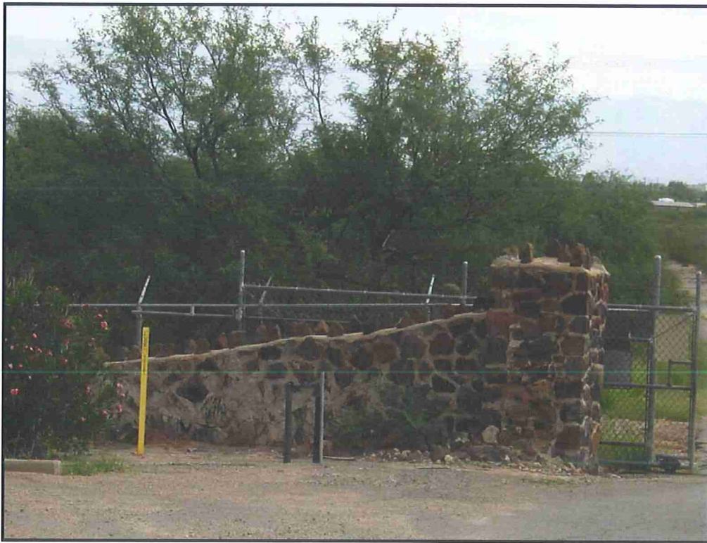
Photograph 46. Volcanic cobble perimeter wall at the former San Xavier Sanatorium, view facing east-southeast (2010).
