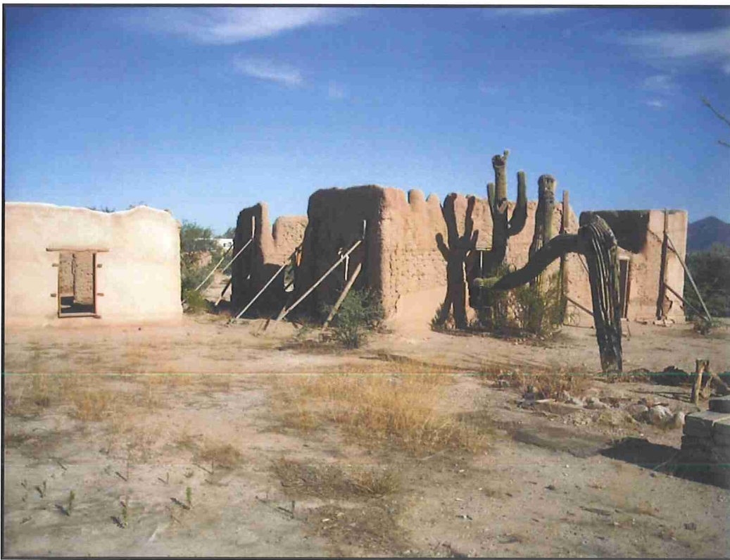
Photograph 34. Remains of Officer's Quarters No. 1 and 2; former Cate's Sanatorium, view facing west-northwest (2010).
